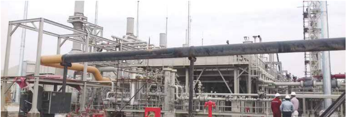
For achieving desired pressure: Installation of compressors in progress at HQ-2 Daur
