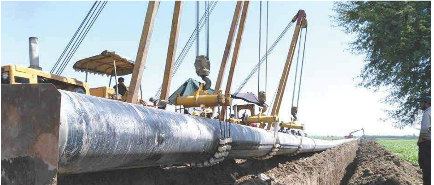
Total Commitment: Work on RLNG project in full swing in Lower Sindh
