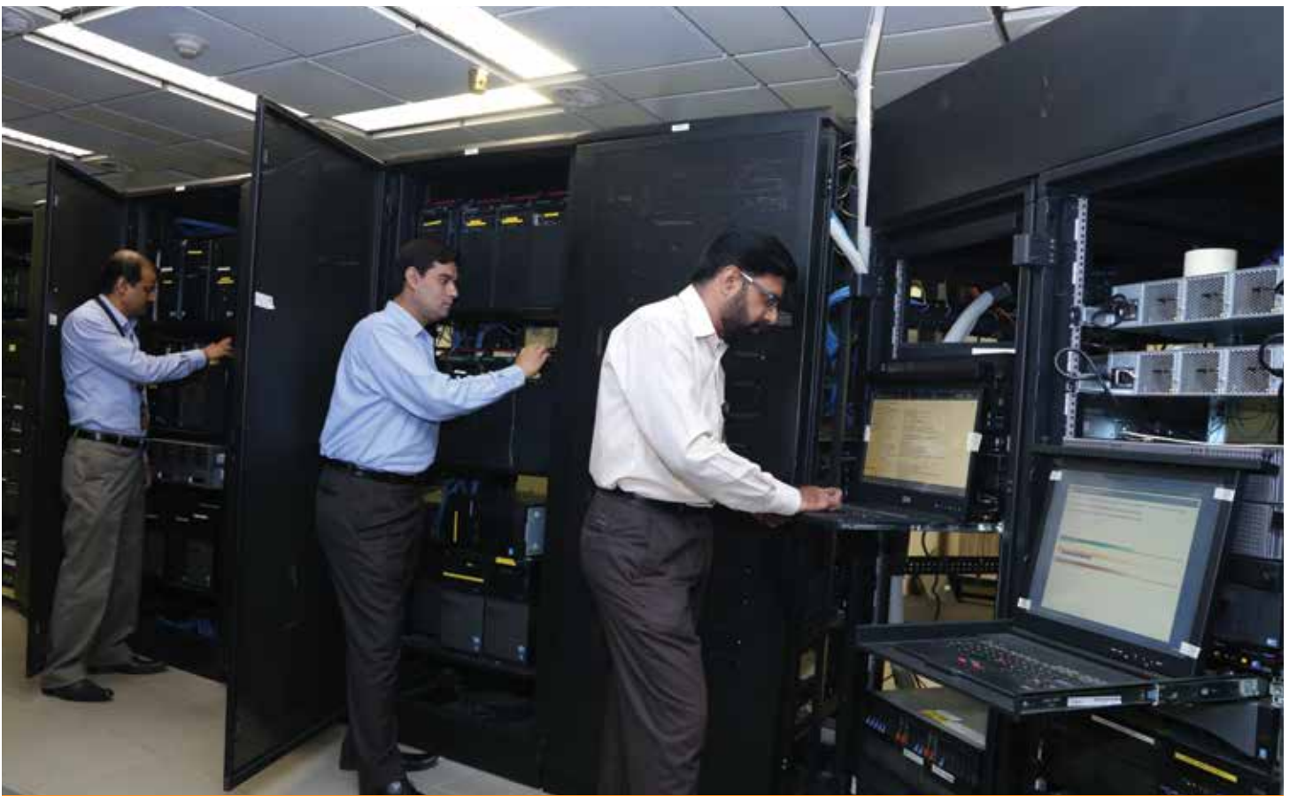
Men at work: Company's IT professionals at work in the main server room
