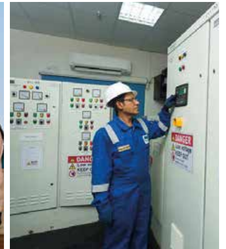
Sync panel - Sujawal MCC
