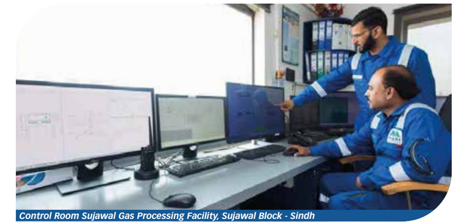
Control Room Sujawal Gas Processing Facility, Sujawal Block - Sindh
