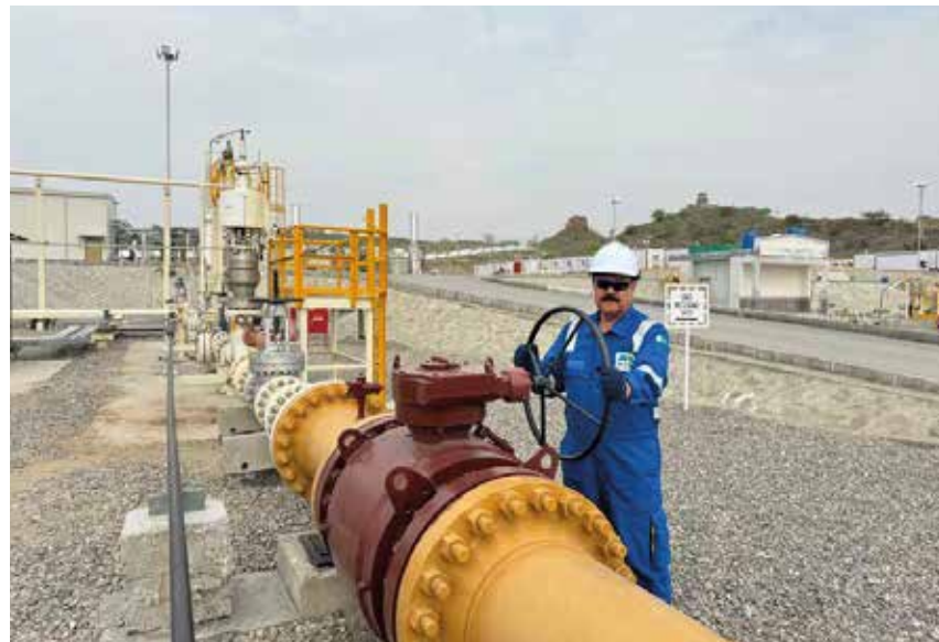
First Gas Production, Waziristan Block - KP
