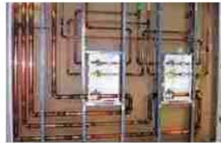
Medical Gas Pipeline
