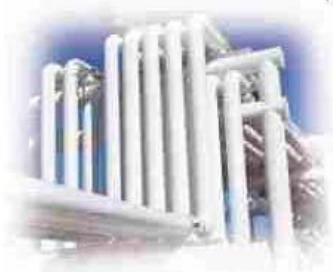
Industrial Gases Pipeline
