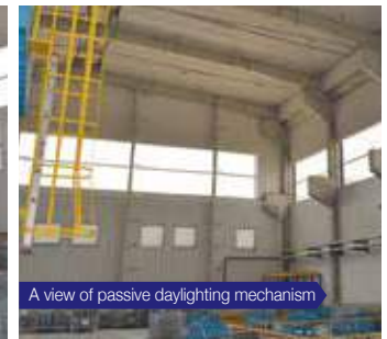
A view of passive daylighting mechanism
