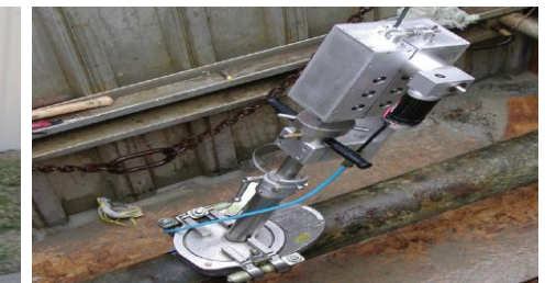
Gas Theft Detection- Inline Camera
