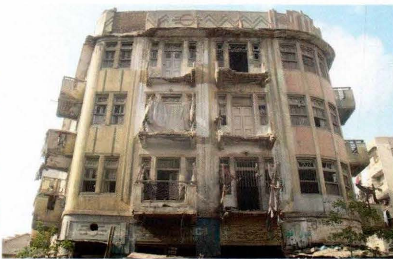
KARACHI: A decaying building at Ath Chowk needs attention of authorities. -Online
