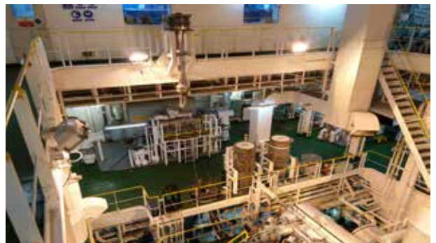
Engine room of M.T. Khairpur
