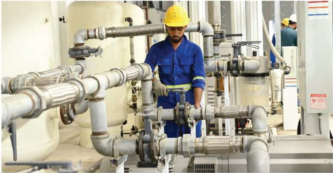
World's largest medical air plant supplied and installed by Pakistan Oxygen at a prestigious hospital in Karachi.
